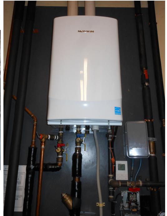
Navien High-Efficiency Gas Water Heater with Recirculation Loop on the former Gregg School
