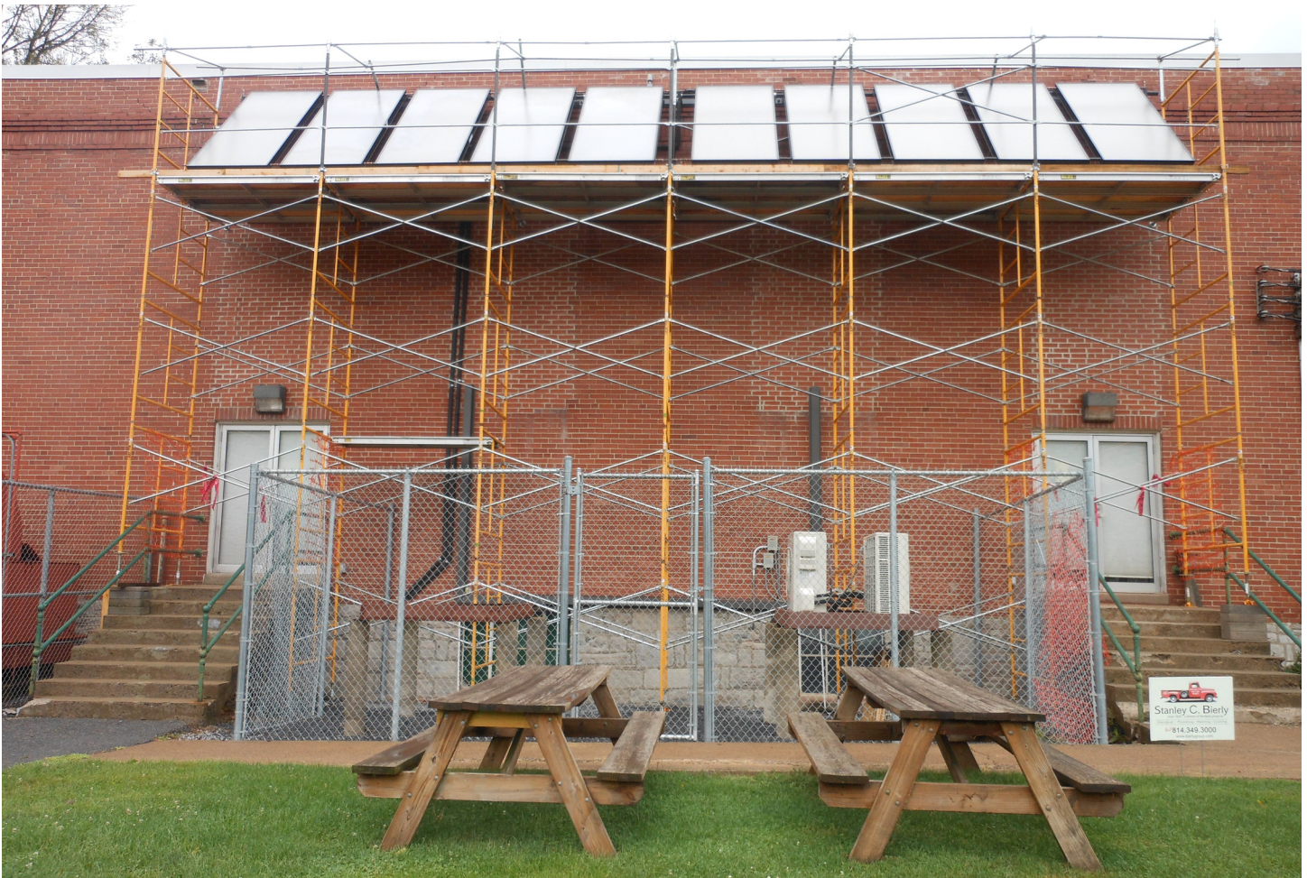
Viessmann ten-panel Solar Domestic Hot Water System mounted on the south-facing gymnasium wall. (Photos by Curt Bierly)
