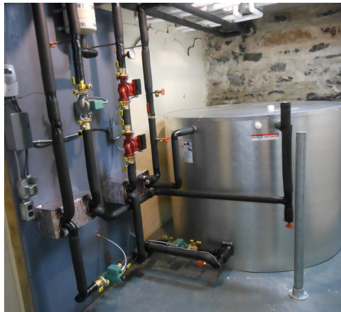
Insulated Solar Tank and associated Controller / Circulators / Heat Exchangers
