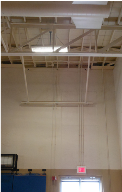
Structural 'kickers' designed to protect the south gymnasium wall against snow and wind load on the panels
