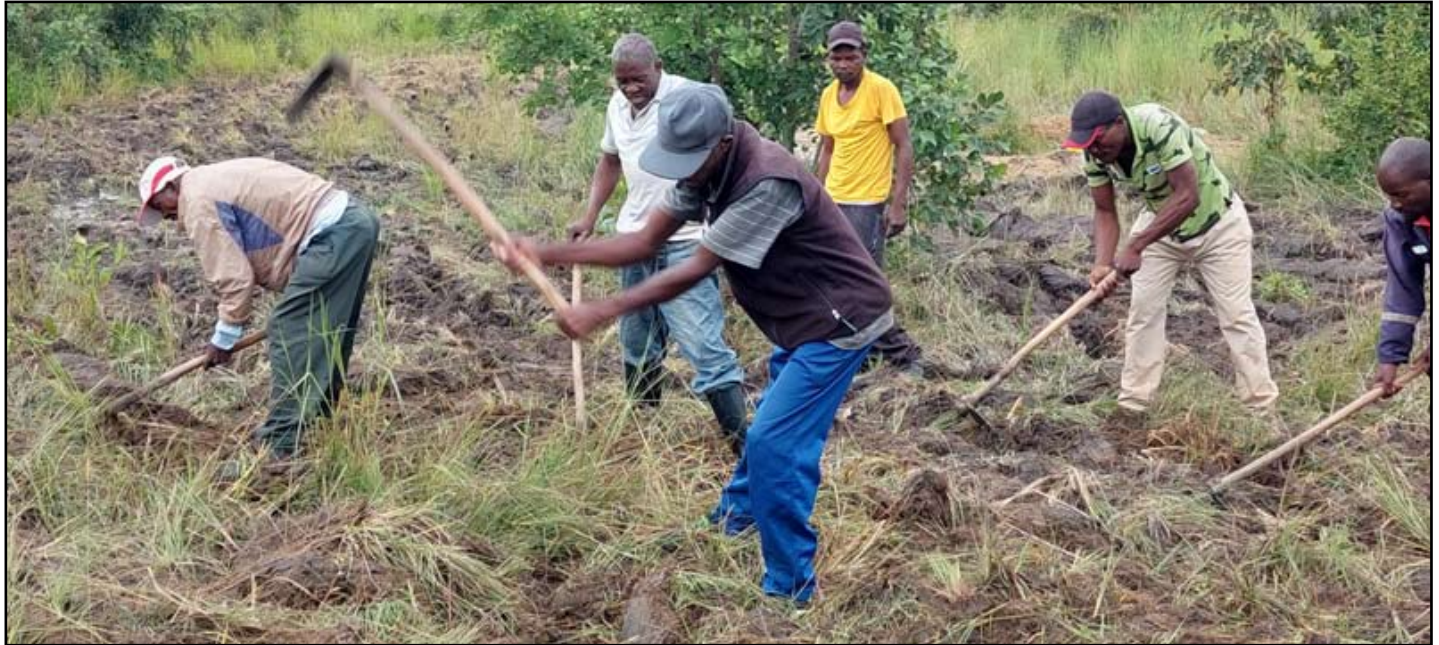
Workers till the site of the new garden at the permaculture site.
