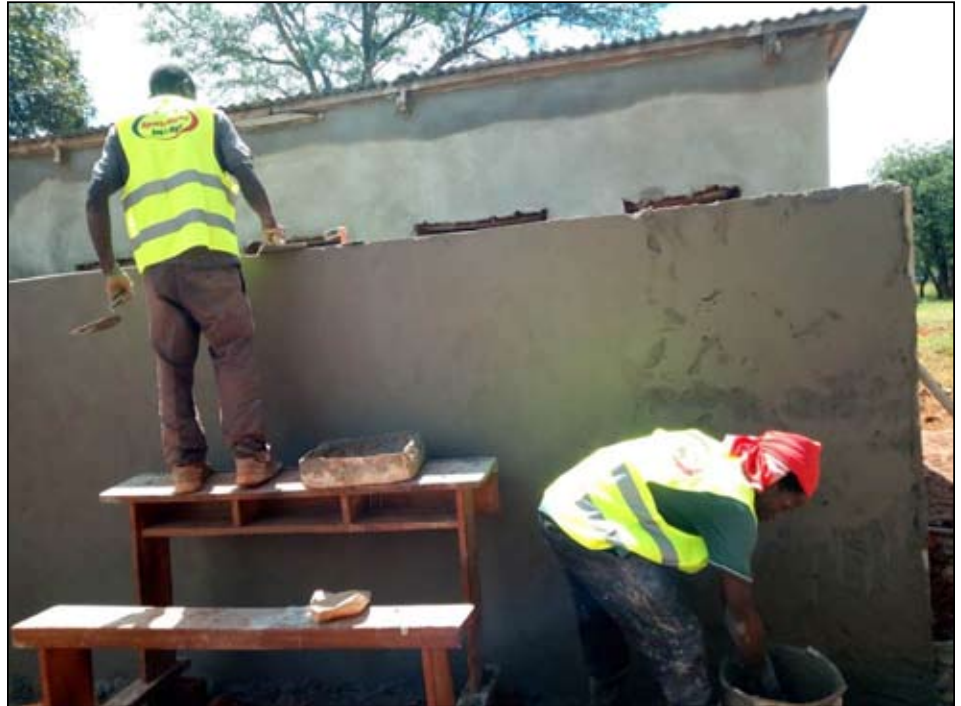
The renovation we have started with the support of the U.S.-based organization Sports Works International NGO. Sports World International. This photo shows the workers plastering the outer walls of the girls' washroom in a primary school.
