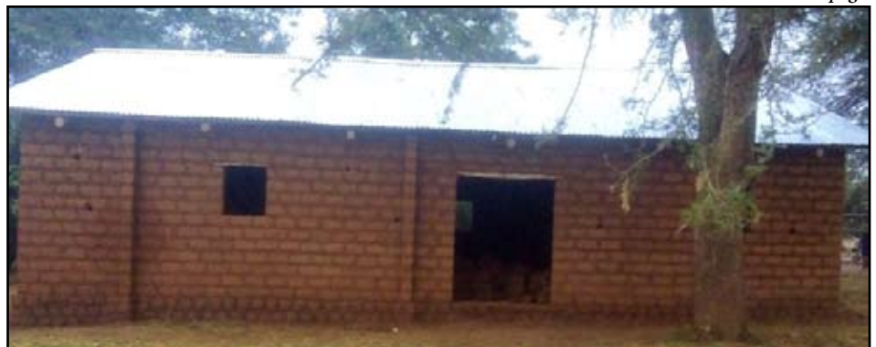
This is the current level of the building that needs finishing. If New Hope for All raises $800, they can buy windows, doors, sand, cement, and labor so that it becomes useful.
