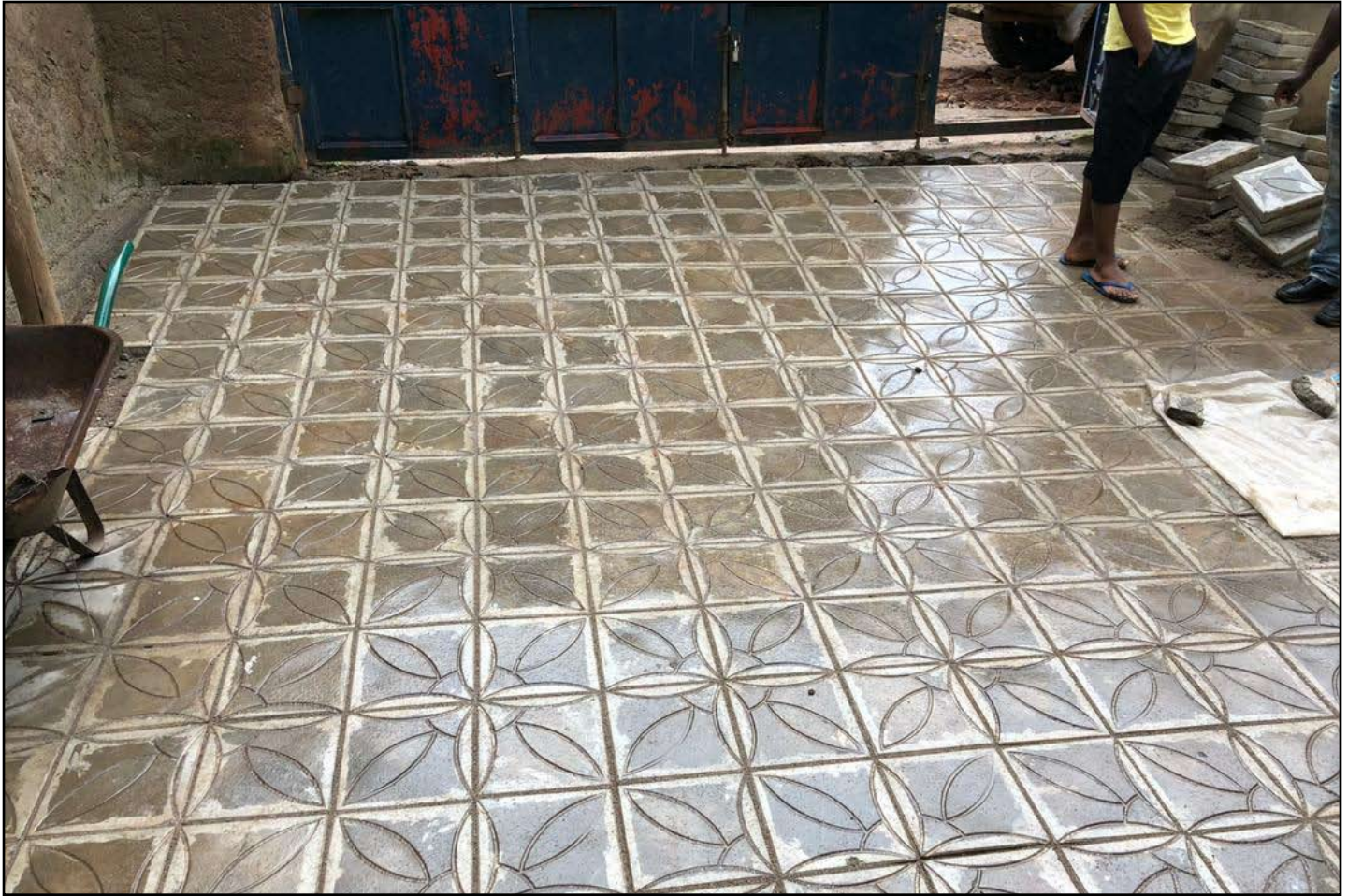
Photos Courtesy A.S.E.
