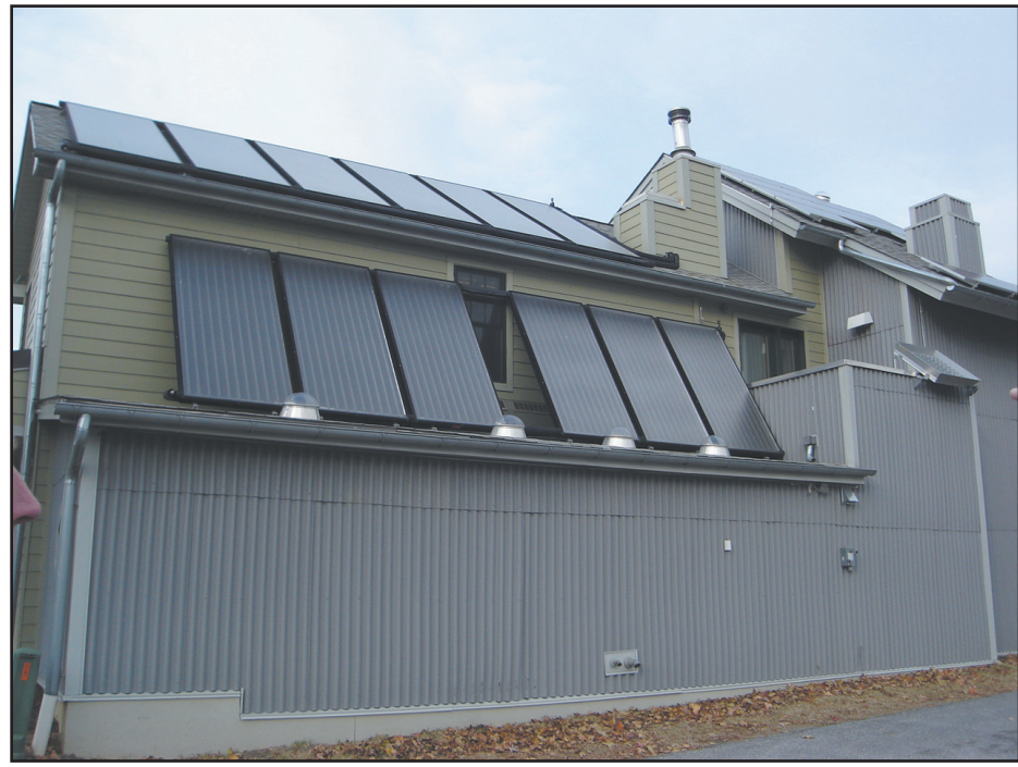
The public was invited to visit the EnviroCenter in Jessup MD on December 2 to learn about "Building a Green Economy." Executive Director David Woolley-Wilson (right) gave "The Order of the Earth" a special tour. This side view of the building showing photovoltaic and thermal solar panels, which provide electricity and heat. The gray siding is recycled asphalt shingles. Photo by Iona
