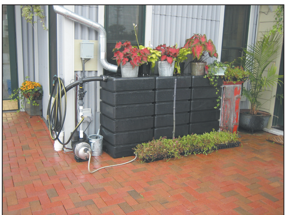
Nothing goes to waste here. Rainwater from the roof is collected and drips into Rain Boxes (see also rain barrel story on page 14). Then it travels through special irrigation tubes to water plants in the garden or pots. Photo supplied by GBI
