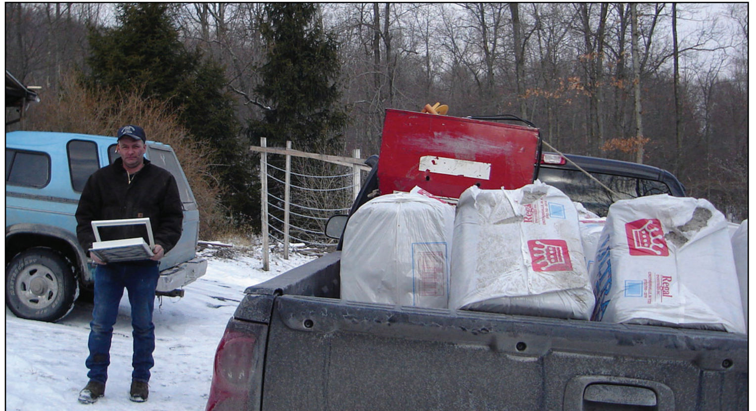
Paul Smith organized the work. Here he is shown with a truckload of paper insulation for the attic. He also replaced three thermostats, a fan and a basement baseboard heater that was coming on sporadically, wasting energy in summer as well as winter.
