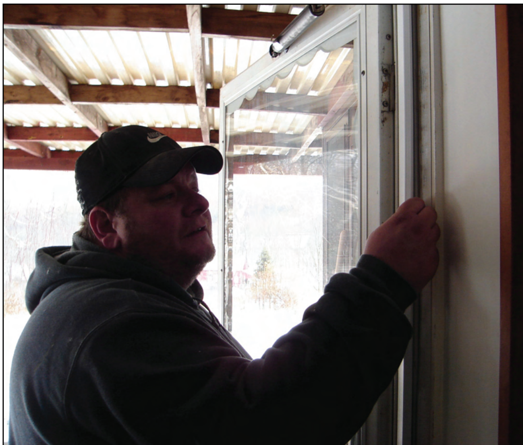
John Wilson worked hard to seal up our basement door. He put foam-filled weather-stripping around the door and a "sweeper" at the bottom to prevent cold air from coming in. He also plugged up our dryer vent since we will never own a dryer and a lot of cold air was coming in through it. It had been "out of sight and out of mind" during all our earlier efforts.
